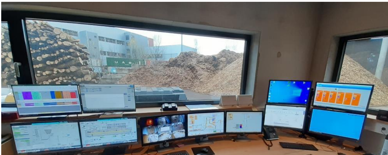
Figure 5.24 Control room of a biomass CHP plant (source: AEE INTEC).
