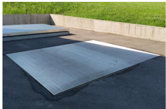
Figure 6.9 Silo lid not accessible in the background and accessible in the foreground. Both in closed condition. (Source: Schmid energy solutions).
