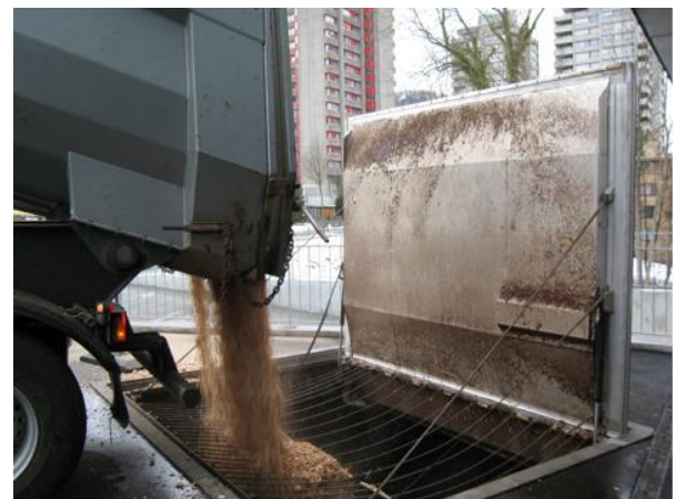
Figure 14.1 Feeding the underfloor silo (source Holzenergie Schweiz).
