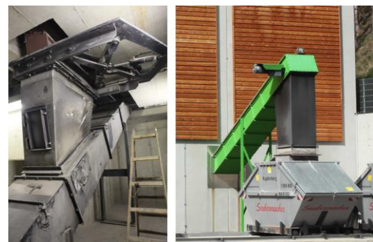
Figure 6.41 Mechanical ash removal conveyor: with scraper chain conveyor (source: AEE INTEC).
