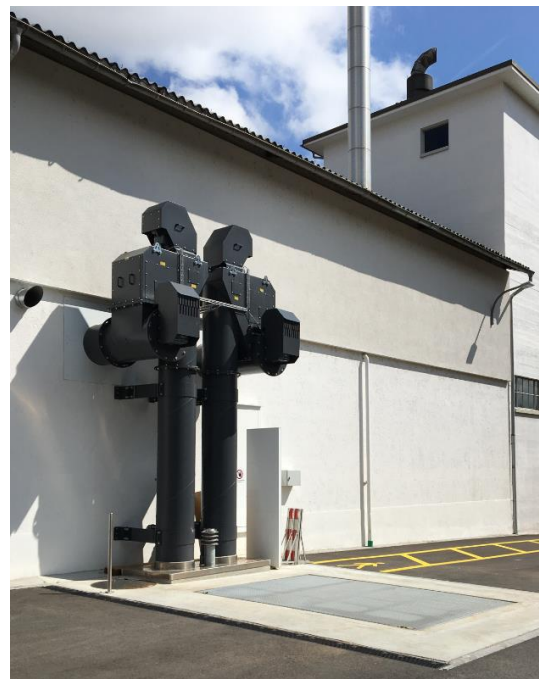
Figure 6.13 Vertical screw conveyor system (source: Schmid energy solutions).
