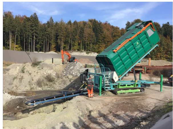
Figure 9.2 Dust-free depositing of wood ash into a landfill (source: Amstutz Holzenergie AG/Holzenergie Schweiz).
