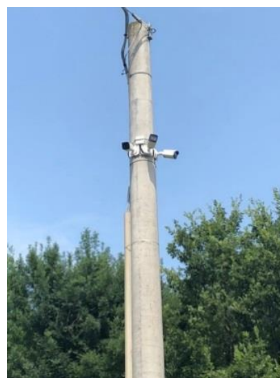
Fig. 24 - Enel concrete pole with the three cameras installed.
