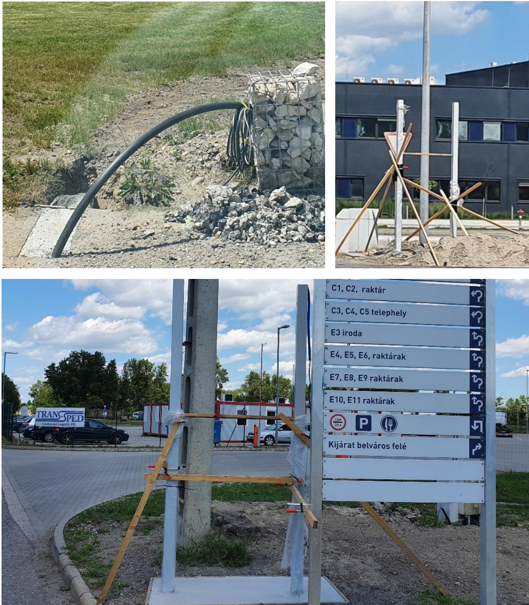
3. Figure: Supplier primer work in order to be able to install hardware on-site of FBL
